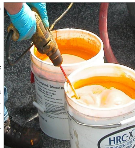
Mixture of injection liquids used to treat groundwater. A single injection at a site can cost from $75,000 to $150,000.
